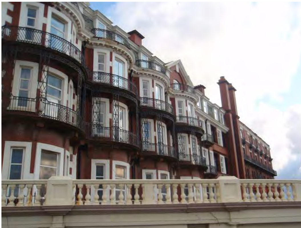
Fig. 27: Early 20 th -century ironwork balconies to the west elevation of the Metropole Hotel
