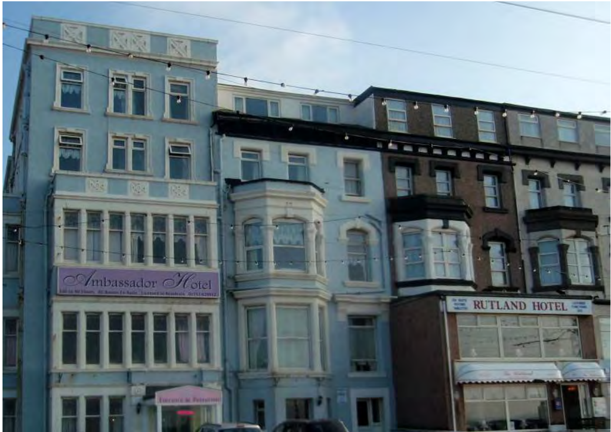
Fig. 19: Sash windows to the square bays of the Ambassador Hotel, and unsympathetic uPVC replacements in the neighbouring building
