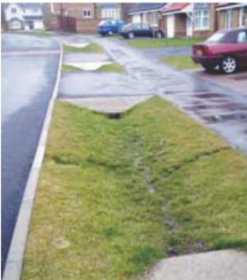
Figure 5 Example of an urban swale - CIRIA C698 'Site handbook for the construction of SUDS' by CIRIA
