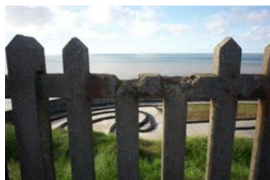
Broken and corroding concrete fencing
