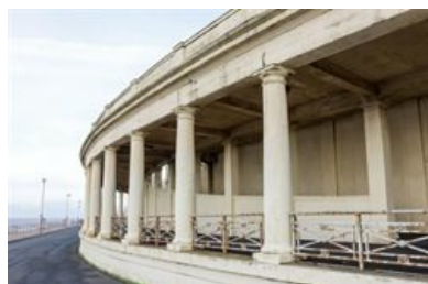
Railings in need of repainting
