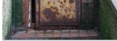
Badly rusting security doors to disused toilets under promenade lift entrance
