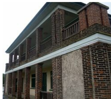
Former disused tennis pavilion which suffers from repeated vandalism
