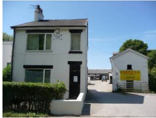
Plate 28. Midgeland Villa built in 1894 with its cart shed to the rear. It has been badly modernised with the loss of its brick façade and traditional sliding sash windows, but it does retain its ridge tiles, datestone and a traditional doorway with overlight
