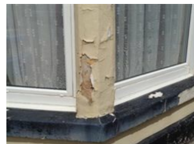
Modern paint traps water which freezes in the stone causing it to crack and flake away.
