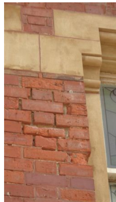
Late Victorian building repointed with cement mortar which has led to front damage.
