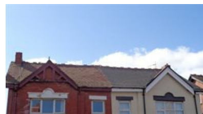
Red clay tile roof covering to the left and modern roof tile to the right of this pair of semi-detached villas.
