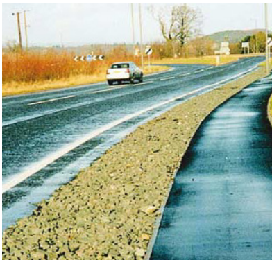
(a) Infiltration trench alongside a road – no kerbs or gullies needed to be incorporated in the design
