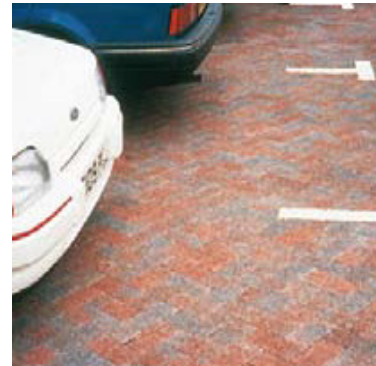
(c) Pervious pavement reduces the risk of surface runoff flooding without compromising on the car park's utility
