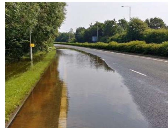
Highway flooding on the A584 in Freckleton 11 August 2020
