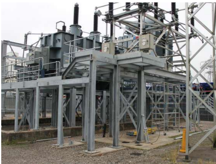
Power Station at Lancaster
