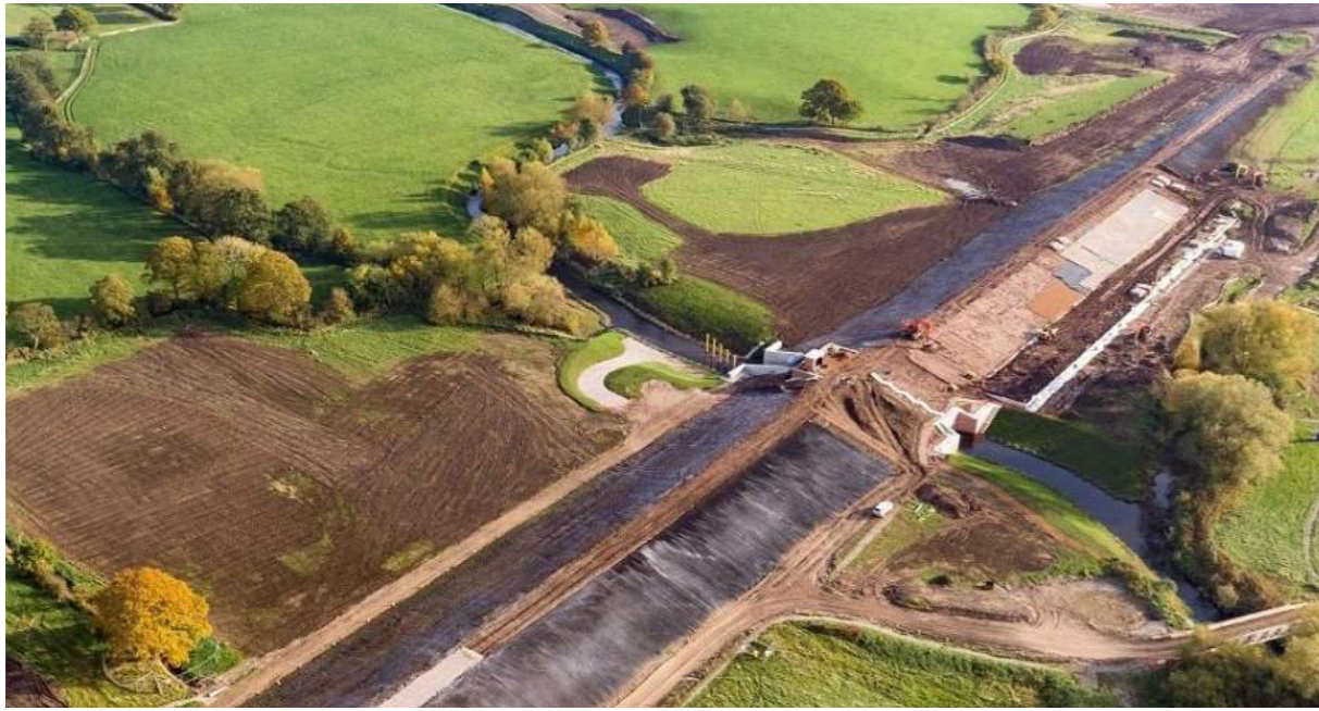
Figure 9: Working in partnership with Lancashire and Chorley Councils “Croston Dam” protects 400 homes and businesses from flooding.
