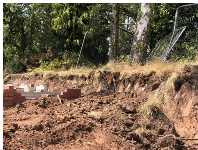
Figure 6: Unacceptable tree protection and site standards, with major structural root damage.
